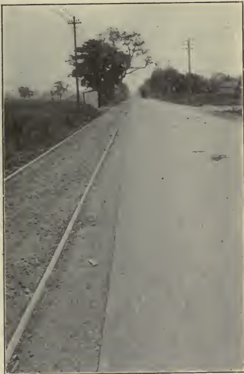
PAVING-GUARD ALONG EDGE OF A HEAVY-TRUCKING THOROUGHFARE IN SOUTH-WEST PHILADELPHIA
